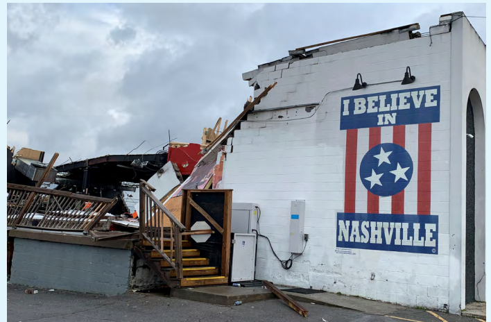
Basement East, a popular music venue in East Nashville, was among the buildings damaged by the tornado
